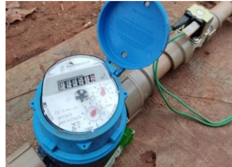
Figure 22 – Water meter at the end of autonomous irrigation (5180 liters).
