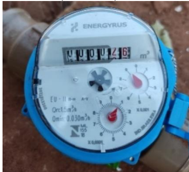
Figure 21 – Water meter at the beginning of autonomous irrigation (260 liters).
