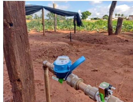
Figure 15 - Water Meter and Solenoid Valve Installed
